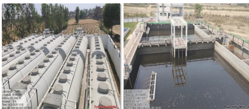
Figures: 10 MLD STP, Kashipur; 500 KLD STP Beljuri
