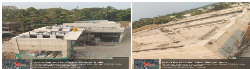
Figure: 30 MLD at Babanpur and 8 MLD STP at Monirampur
